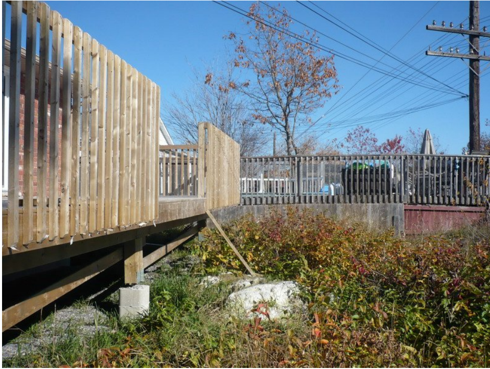
PHOTO 5 953 HOWEY DRIVE, SUDBURY – VIEW OF REAR DECK FACING SWIMMING POOL ON PROPERTY ABUTTING EAST
